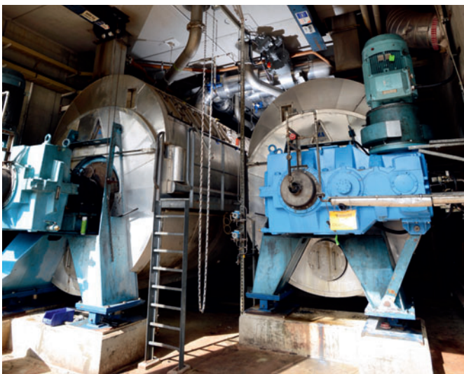
Sludge is concentrated in disc dryers
