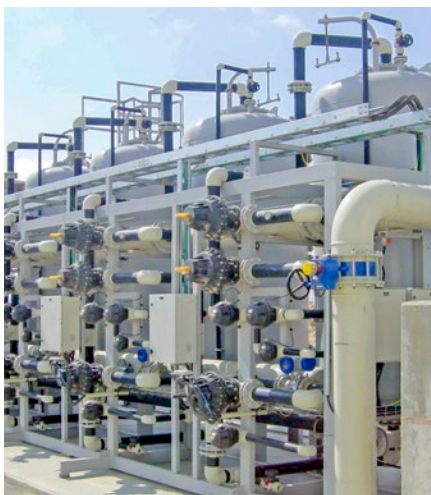
Water treatment (Treitel Chemical Engineering Ltd)
