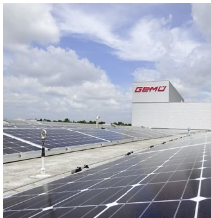
Photovoltaic panels in the European Production and Logistics Centre
