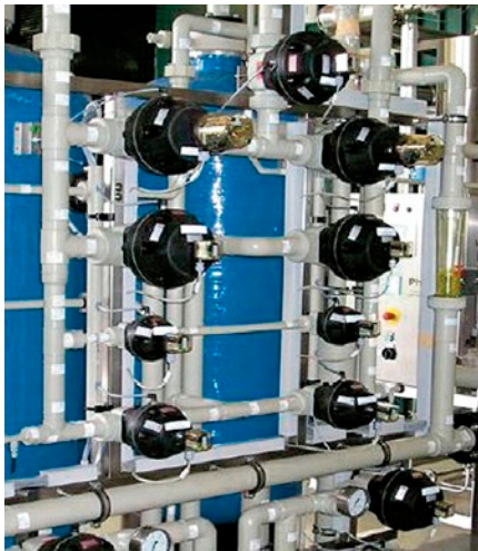
Plant with PP components
