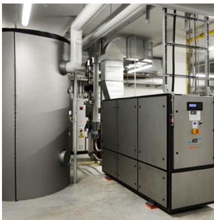
Combined heat and power plant in the European Production and Logistics Centre
