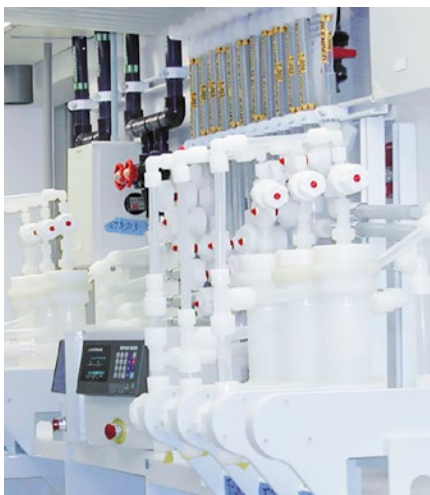
Chemical filling installation
