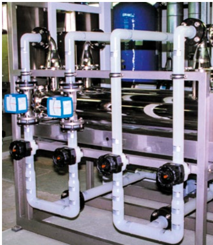
DI water treatment
