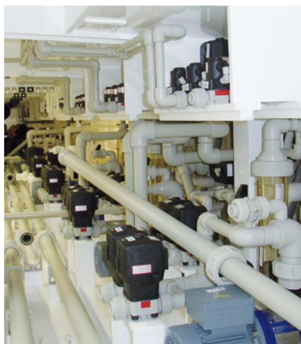
Media area of an etching and cleaning installation
