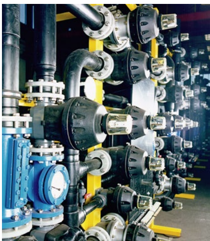
Waste water plant with PVC/PE components
