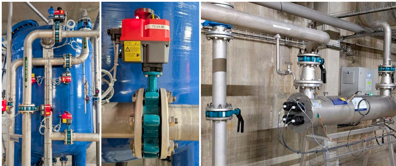
Sand filtration using motorized butterfly valves GEMÜ R488 Victoria and UV disinfection with manual butterfly valves GEMÜ R487 Victoria
